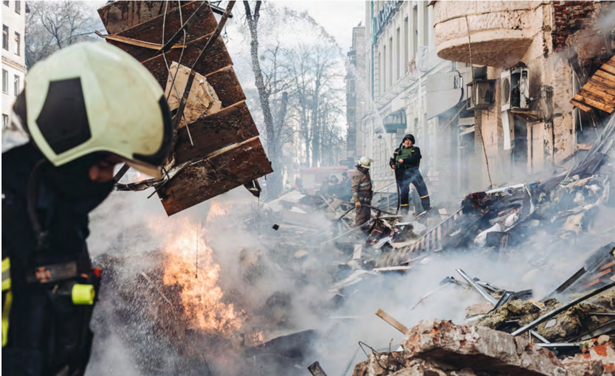
Firefighters work on a building destroyed by a Russian shell, in Kharkov, Ukraine, 14 March 2022. (Diego Herrera Carcedo - Anadolu Agency)
